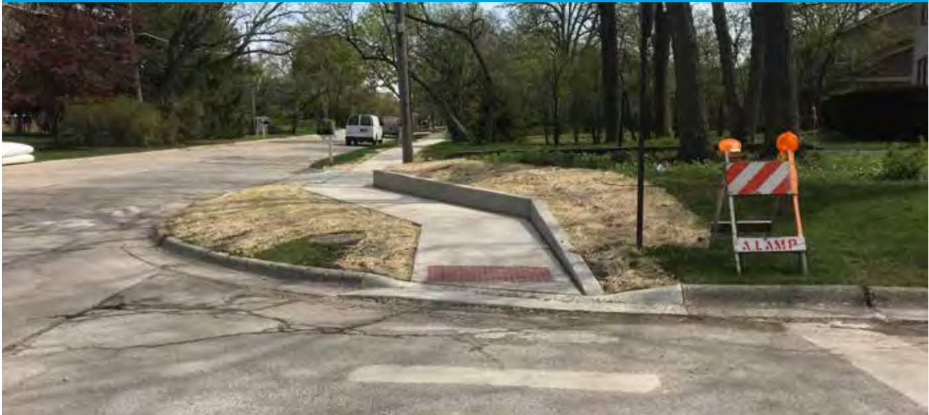
New sidewalk construction in Spring 2019 on Ridge Road, between Lake Cook Road and Lawrence Lane fills a critical gap in the sidewalk network.
