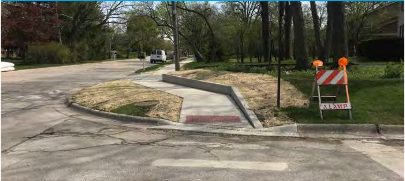
New sidewalk construction in Spring 2019 on Ridge Road, between Lake Cook Road and Lawrence Lane fills a critical gap in the sidewalk network.
